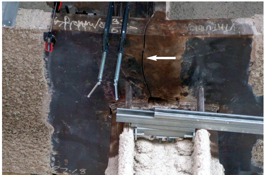
Fig. 3 — Example of brittle fracture at the north girders of the Transbay Transit Center. (Photo courtesy of Transit Joint Powers Authority.)
